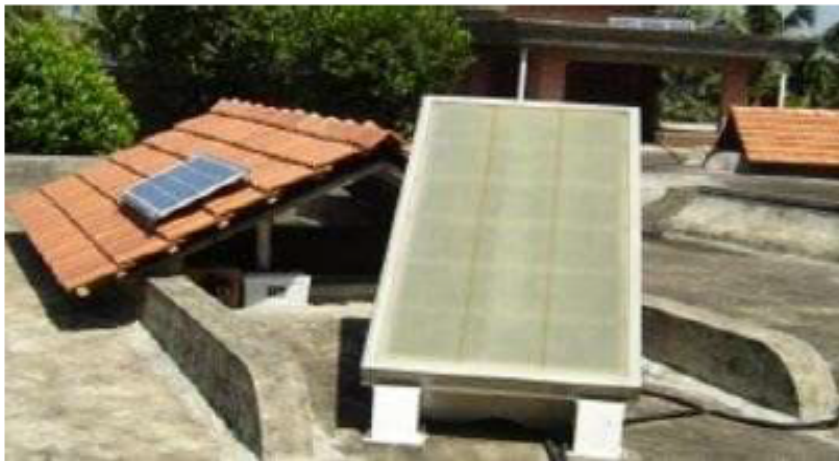
Solar Panels on the roof
